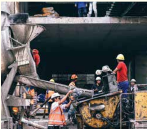
Michigan's prevailing wage law makes public projects more expensive and limits job opportunities for some workers.
