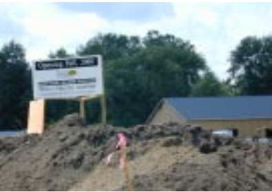
This National Heritage Academy charter school under construction, promises quality education to students in Romulus.
